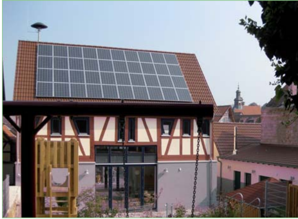
Abb. 39: Private Solaranlage in Nidda
